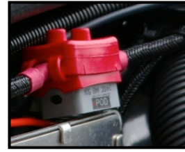
Auto reset circuit breaker
